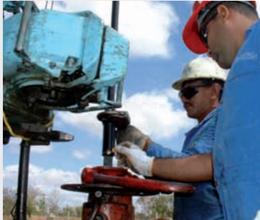
Maintenance of PCP installation
