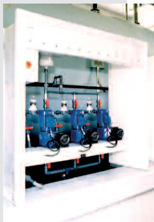
Dosing pumps integrated in a dosing skid for water treatment
