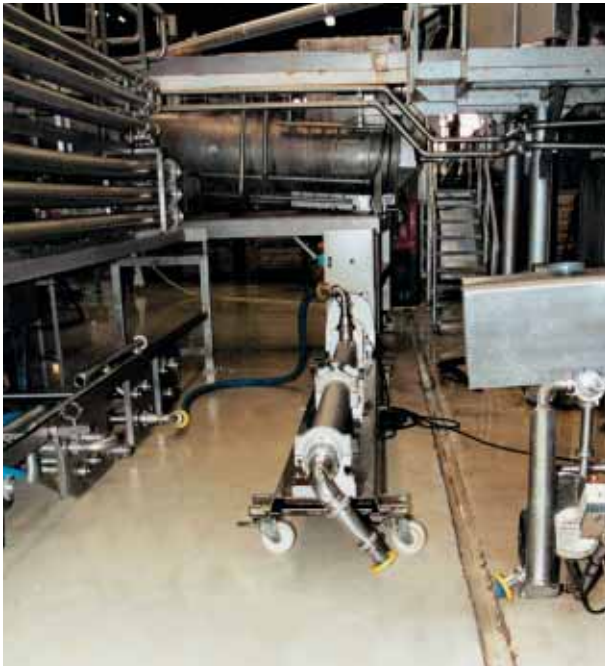
40H24: transformation of fruits and vegetables sector - transfer of fruit purée to an exchanger/cooler.
