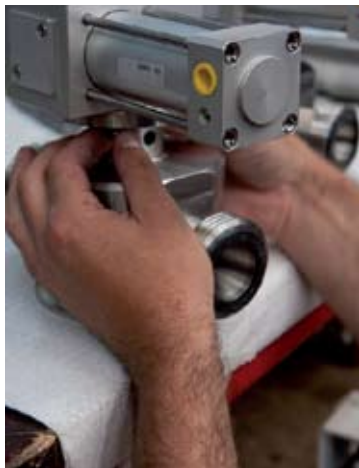
Dosys pump on site maintenance
