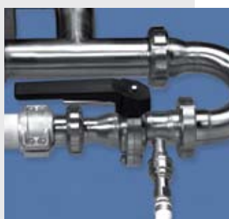
Container suction hose connected to CIP line
